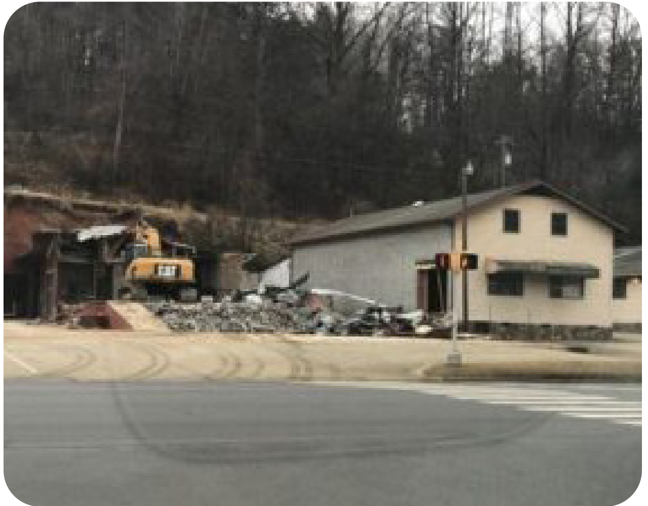
Sylva business Bryson's Farm Supply after more than 50 years had to close its doors once the road work took over. Photo by WCJ.
